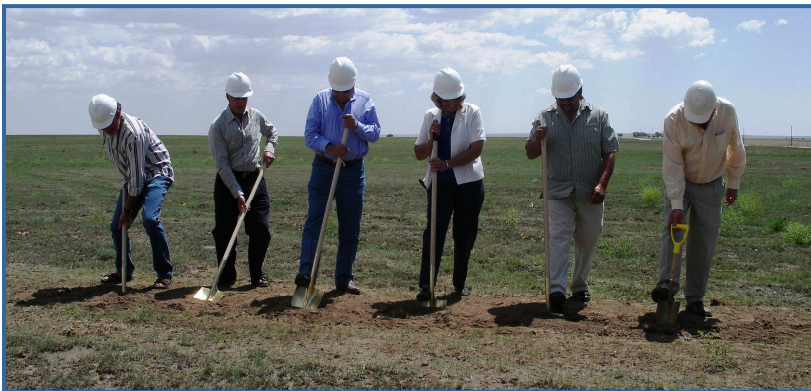
From left: Board Members, Steve Hasbrouck, Andy Anderson, Ted Schubert, Gayle Jones, Robert Lovato and Cherokee General Manager, Kip Petersen, broke ground on the site of Cherokee's new Wastewater Treatment Facility on June 27, 2008.
